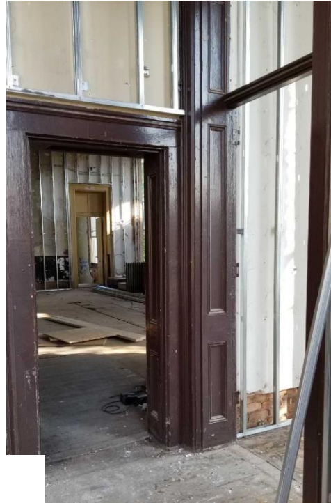
Electrical conduit discovery; the first floor service panel had to be relocated from the first floor to the attic.
